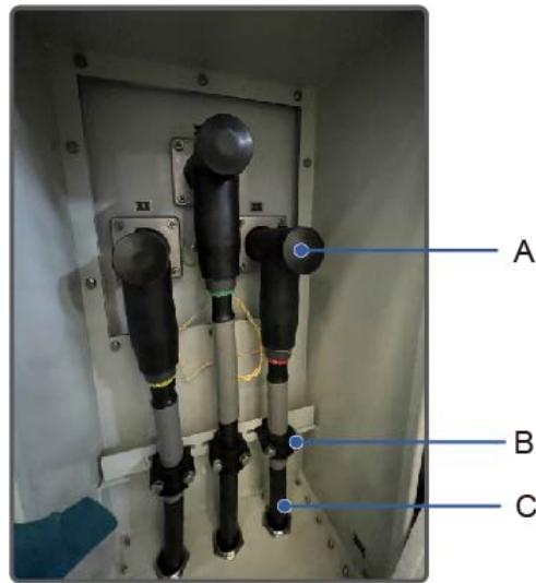
figure 6-5 Cable compartment of the transformer
