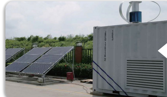
Africa 5 kW/35 kWh Wind and Wind Diesel Storage Micro grid Project
