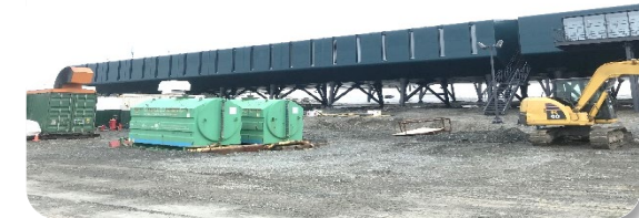
Antarctic Research Station 100 kW/160 kWh Micro grid Project
