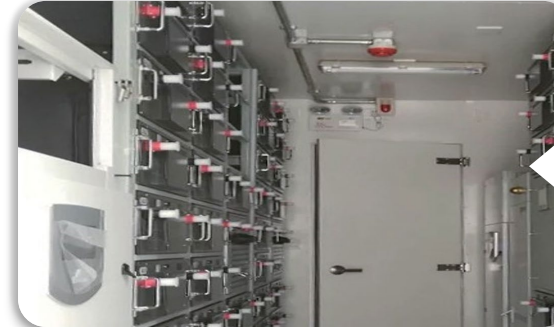
Long Island Substation 500 kW/500 kWh Energy Storage Battery Project
