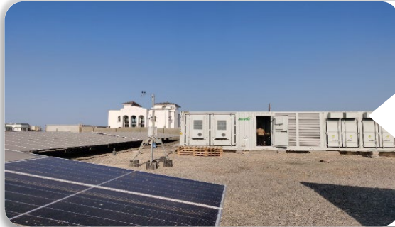
North Africa Gibb 1.14MWh project
